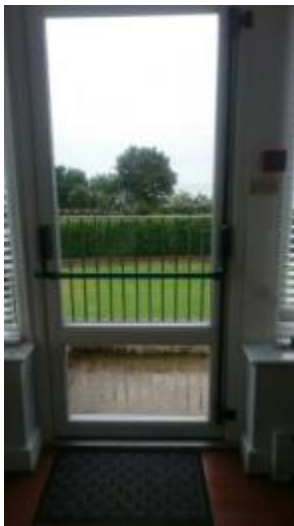
Door from ramp in to restaurant and hotel
